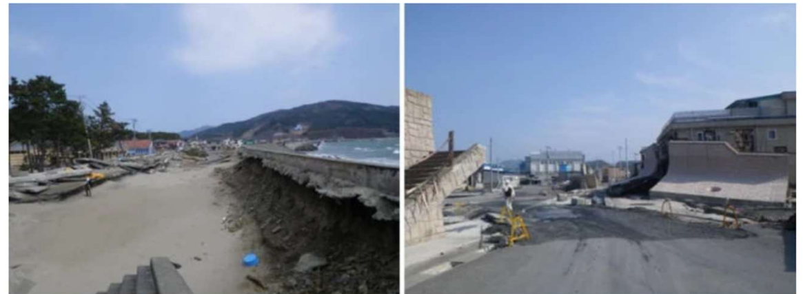
Seawalls damaged by scouring in Ishinomaki city (left, 26/4/2011) and by sliding in Yamada town (right, 31/5/2011)
