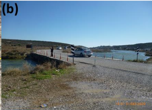
Tsunami traces visible on Alaçatı Azmak bridge
